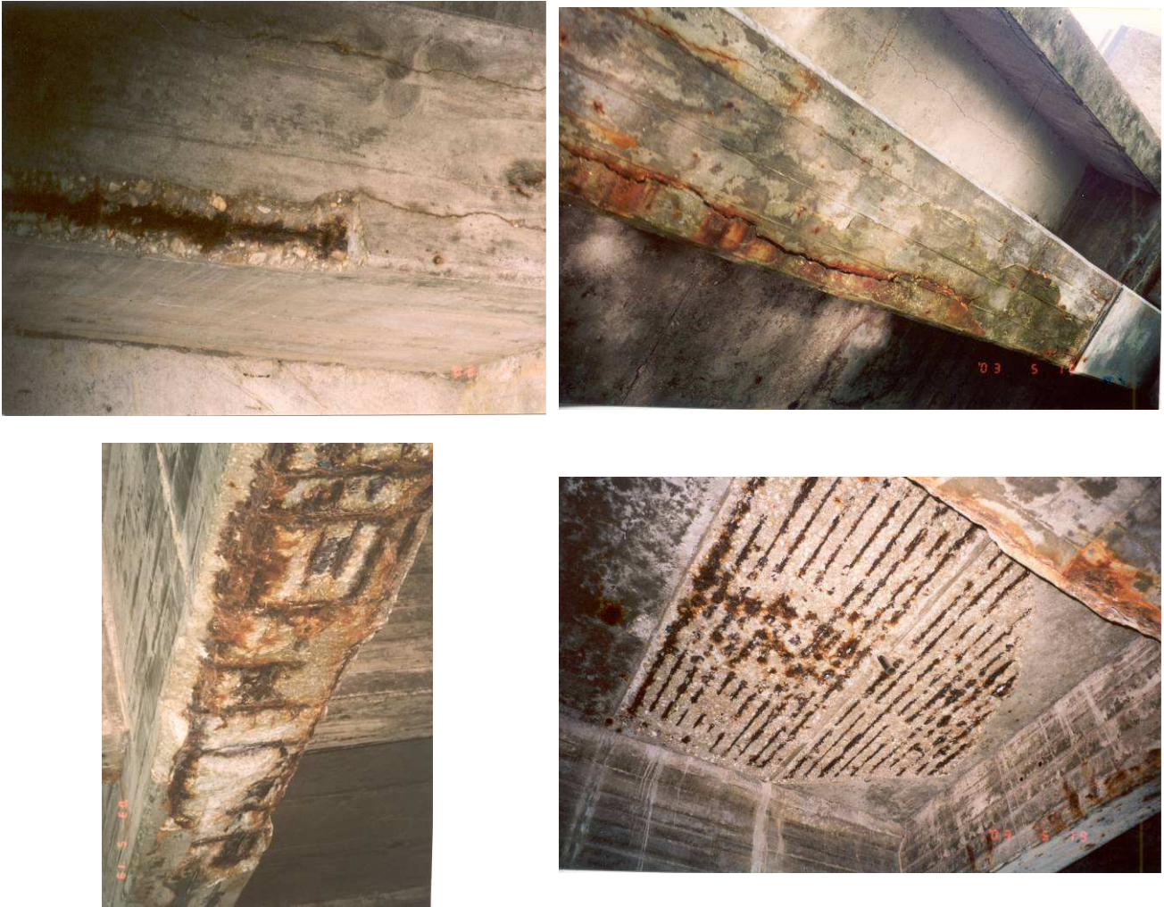
Fig. 3 Deterioration levels in 2004
